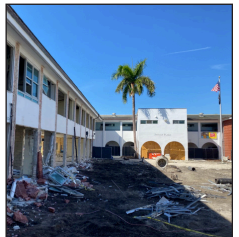
Progress of just under one week of work. (Photo Credit: Ignacio Chazarreta)
